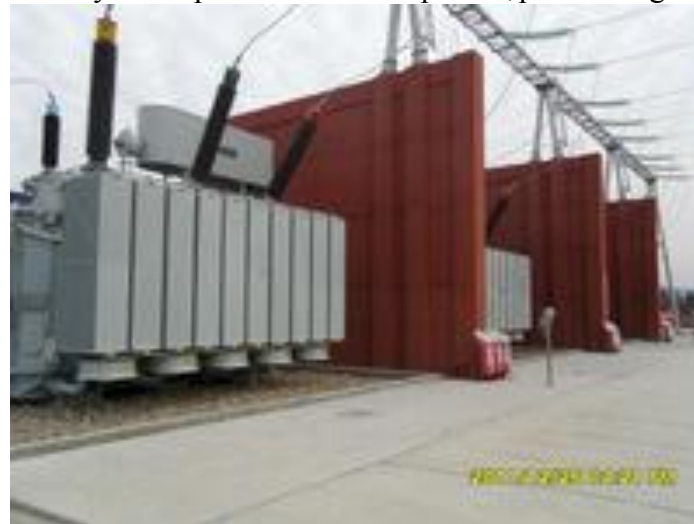
220 kV impedance matching power transformer
